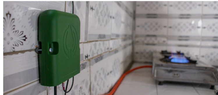
A Smart Biogas node installed near Arusha, Tanzania.
